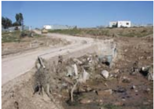
Dirt clogging the sewage passage at the entrance to Um-Batin
