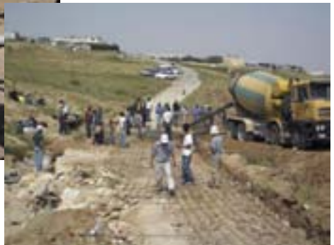
Jewish and Arab-Bedouin volunteer building a bridge together, Um Al-Haran, April 2005 Photo by NCF
