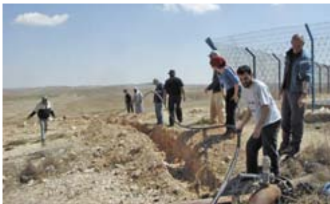
Giving a hand to pull a drinking water pipe line to an unrecognized village.
